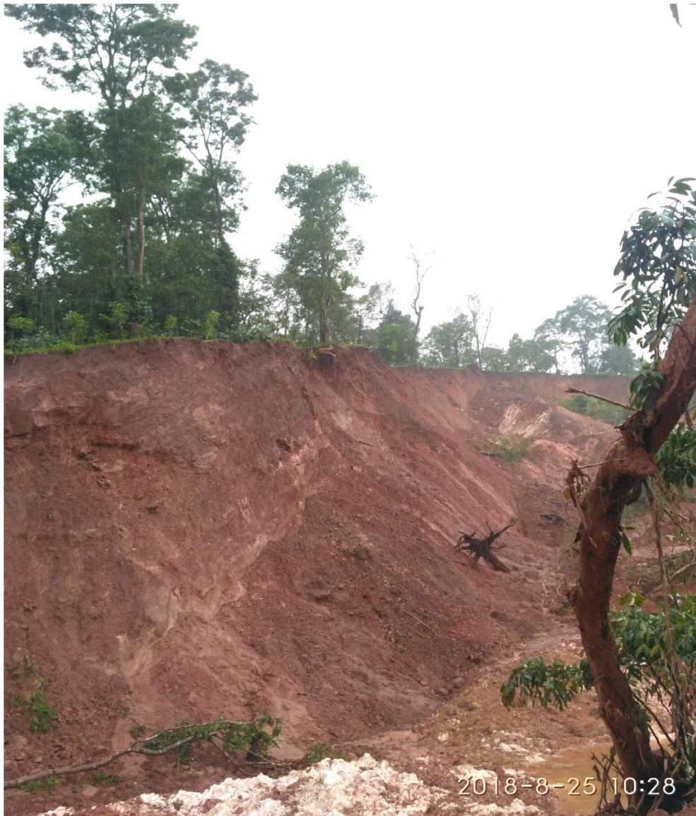
Fig. 2 Landslide Triggerred off by the August 2018 Rainfall Event in Hattihole Region, Kodagu
